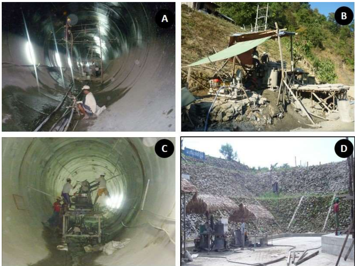
Fig. (4) Grouting along the headrace tunnel: (A) Contact grouting, (B) Grouting machine in the outside area, (C) Consolidation grouting, (D) Grouting machine in the outside area.
